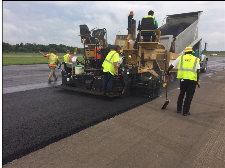
Mill and overlay project for Runway 9R/27L at SBN Source: Mead & Hunt, Inc.
